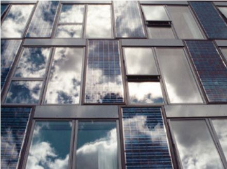
Solceller i facade
